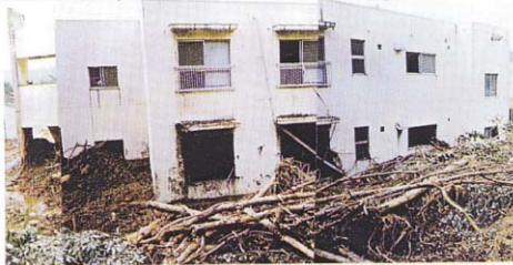
Photo-2 A debris flow that occurred at a hill behind a social welfare facility directly hit the facility, claiming 5 lives (Fukushima Prefecture). (August 27, 1998)
