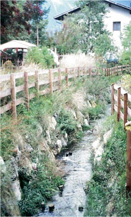
Fig. 4: Channelwork controlling a small flood creek in a settled area. The stream bottom is fixed by low sills as shown in Fig. 2, the banks are protected by walls made of dry-laid stones.
