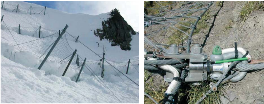
Fig.5: Left: Monitored snow net system in Flaine (74, France) Right: Monitored anchor of the net system
