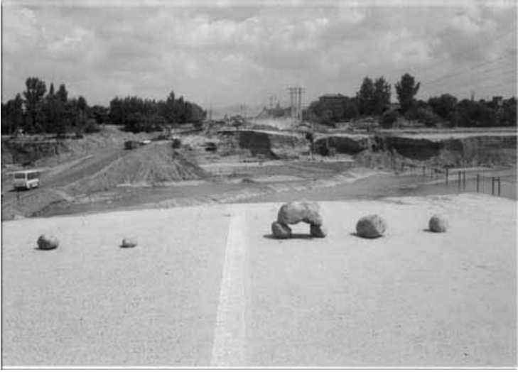
Picture 6 Washed out bridge constructed on main road
