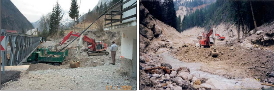
Fig. 11., 12: The Enterprise for Torrent Control removes debris from deposition area (Photo: A. Horvat)
