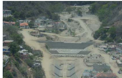
Fig5: Dam and channeling, torrent San José de Galipán. 2003. (Source: CORPOVARGAS)
