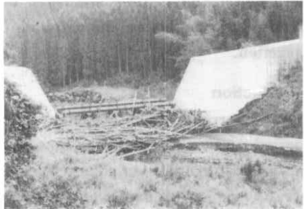
Photo.2 Wood-debris entrapment facility (the upper-stream)
